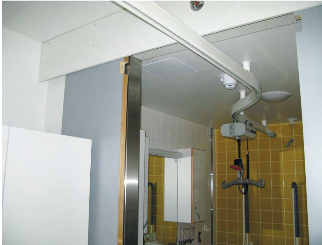
Figure 7. A ceiling lift in a private flat of an assisted living building.
