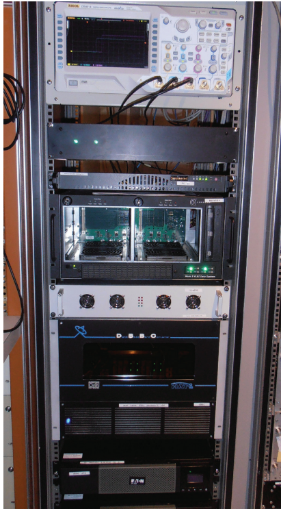
Figure 1.5. The digital VLBI-rack: oscilloscope to monitor the pps-signal, IF-amplifying box, Field System computer, Mark5B+, FILA10G, dBBC and UPS (from up to down).
