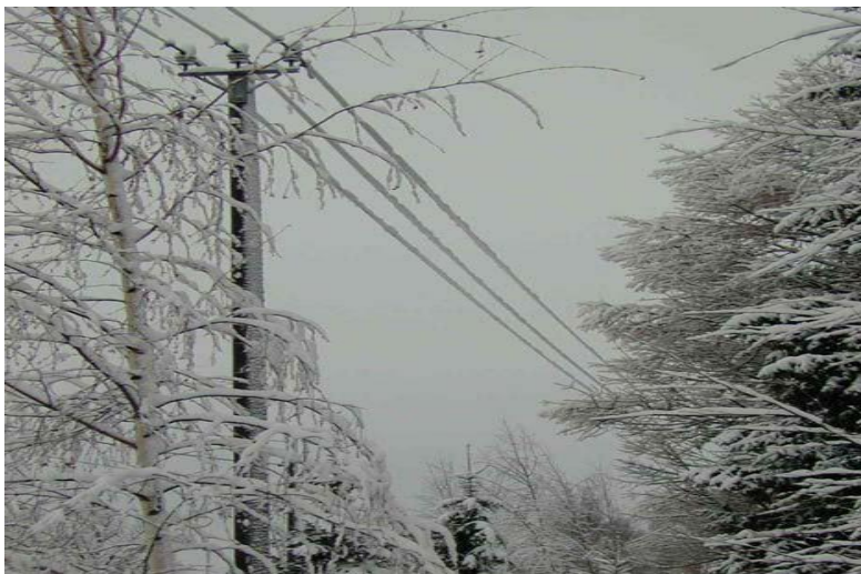
Fig. 1.3 MV covered-conductor lines covered with snow during winter in Finland [1].
