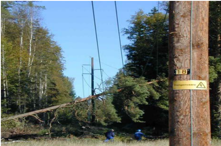
Fig. 1.4 Leaning trees on covered conductor lines in Forest–Sax Line [1].
