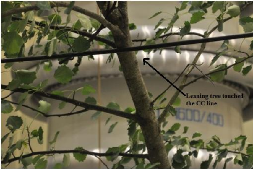
Fig. 5.5 (a), (b), (c) Experimental measurement set-up for PD detection and location resulting from a tree leaning on the CC line.
