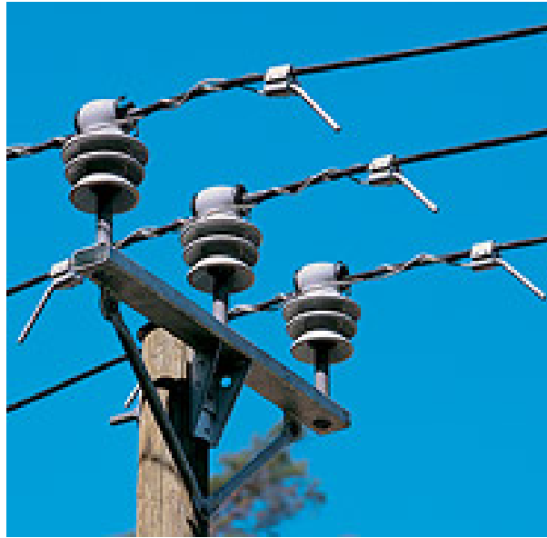
Fig. 2.2 Construction of a typical PAS line – Suspension pole with pin insulators and lightning protection using APDs implemented with arcing horns [13]
