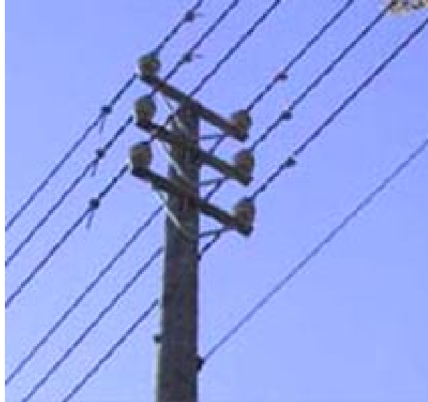
Fig. 2.4 Double 20 kV PAS line – no wider than a normal single bare copper line
