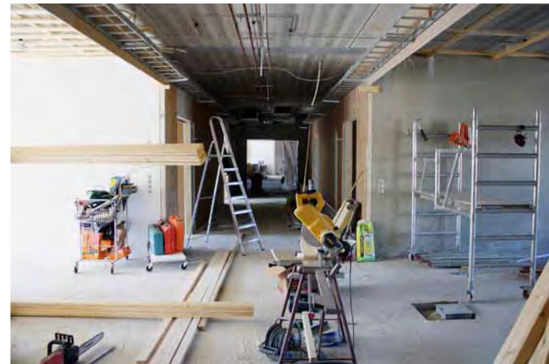
Solängen intensive nursing home. The building process started in October 2010 and was finished in December 2011.
