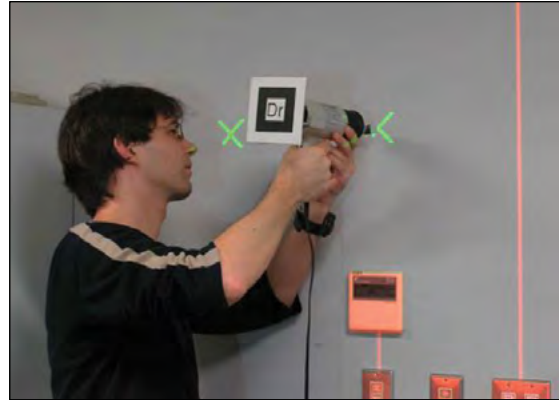
Figure 13: Drill-Guide: This example shows the user where to drill holes and where it's dangerous because of cables [19].
