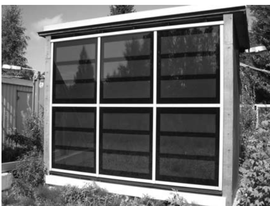
Figure 5.3: a-Si BIPV facade at the HUT test site, with 18 modules.
