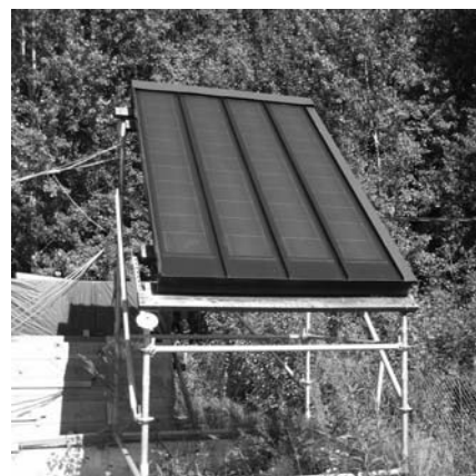
Figure 5.4: Four a-Si modules integrated to a free-standing roof at the HUT test site.
