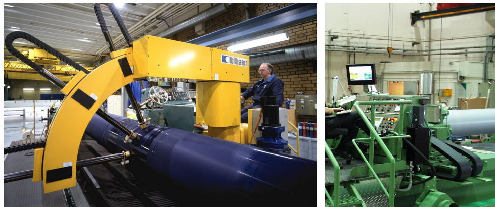
Figure 22 Four-point measuring device (left) and high-precision positioning unit (right) installed in an old roll grinding machine.
