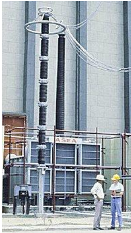
Figure 2.9 Oil-insulated smoothing reactor in the Rihand – Dehli HVDC transmission [32]
