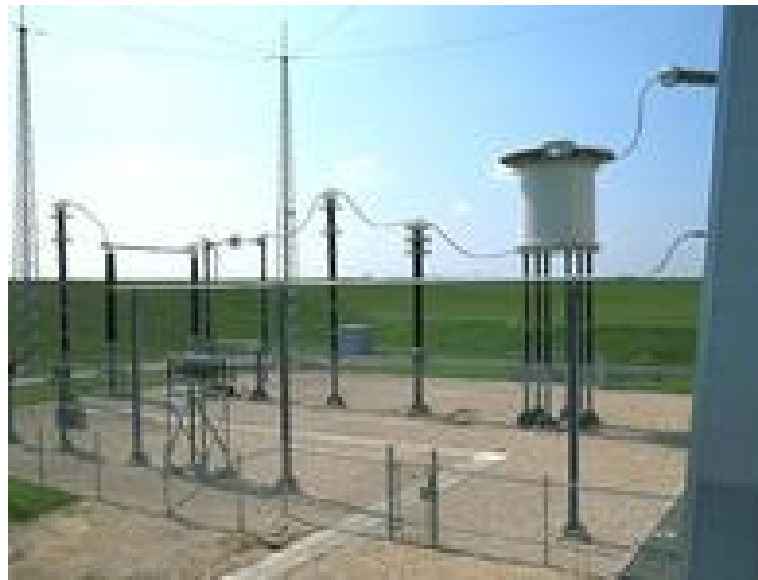
Figure 2.8 Air-core smoothing reactor in the Kontek HVDC transmission [32]
