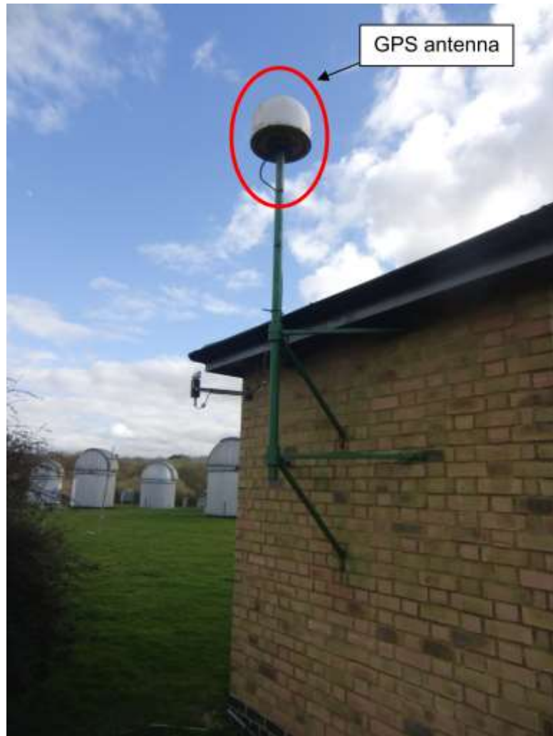
Figure 3-14: Observatory of Bayfordbury, GPS station attached to the hut by a rigid steel frame.
