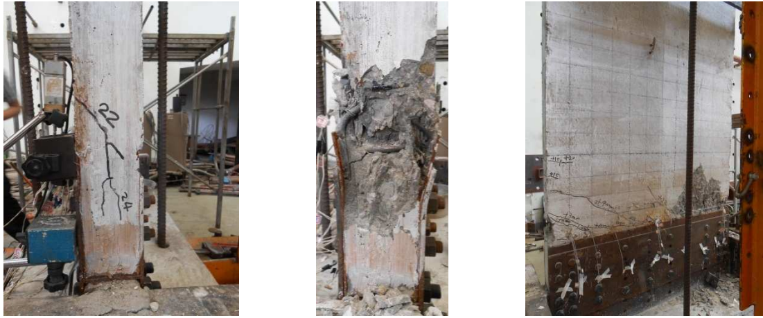
(a) Vertical cracks at compression end (b) Compressive failure (c) Overall failure mode
