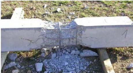
(a) Local damage of RC due to close-in blast [Gebbeken, 2006]
