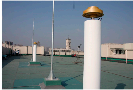
Figure 3. GNSS reference stations in UNNC.
