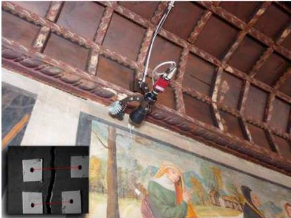
Figure 2-10 Cracks monitoring technique in the Sala dei Battuti – Conegliano Cathedral (Lorenzoni et al., 2016).
