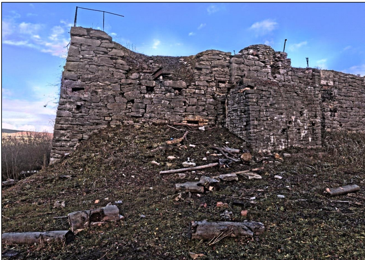
Figure 8-11 Some fallen parts in the SE face.
