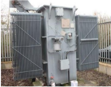
Figure 1: Liverpool Road Primary Transformer
