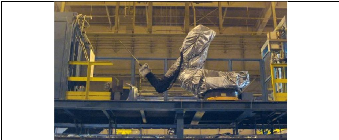
Figure 2-2: LiquiRob installed at LOP for sampling in continuous casting of steel slab (Juergen Meisel, 2014)
