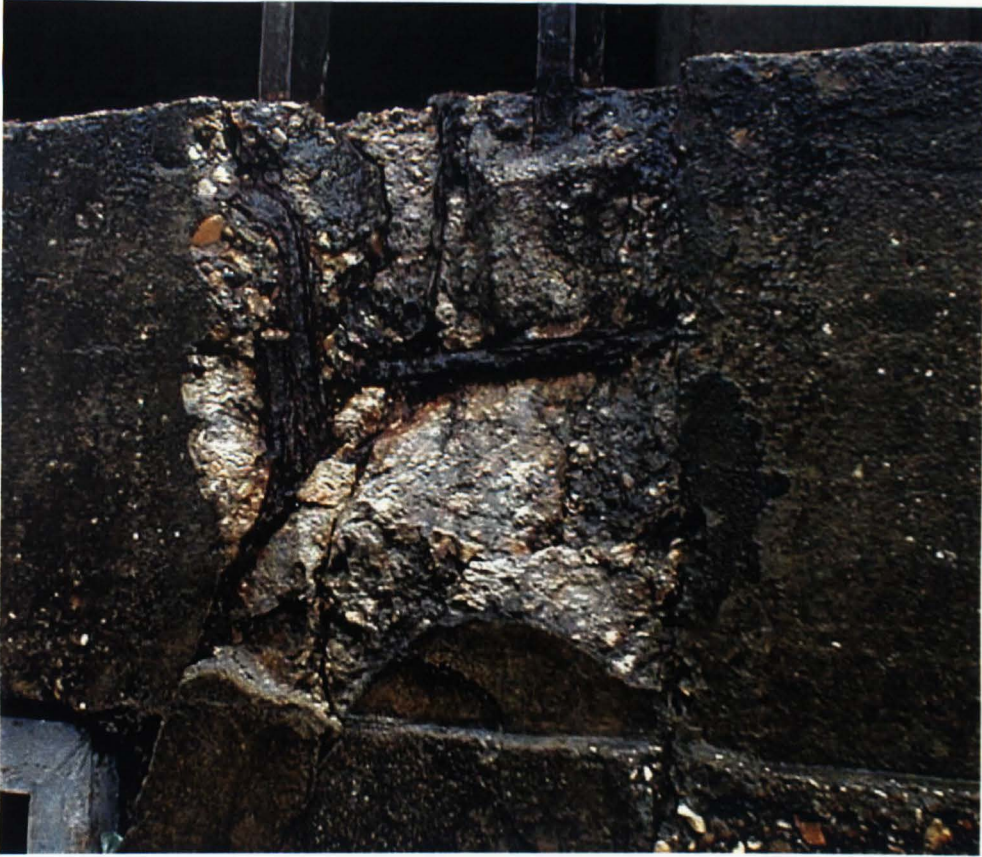
Figure 3-7 Example of spalling due to the corrosion of steel reinforcement.
