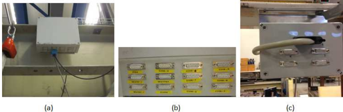
Figure 3.10. (a) Connection box for cone resistance and pore pressure transducers from the bucket foundation, (b) signed sockets on the connection box, and (c) Connection box for the pore pressure transducers from the beam
