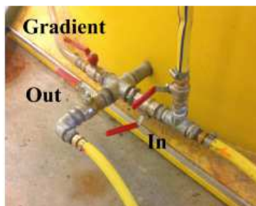
Figure 3.4. Valves controlling the incoming and the outgoing water supply of the yellow sandbox
