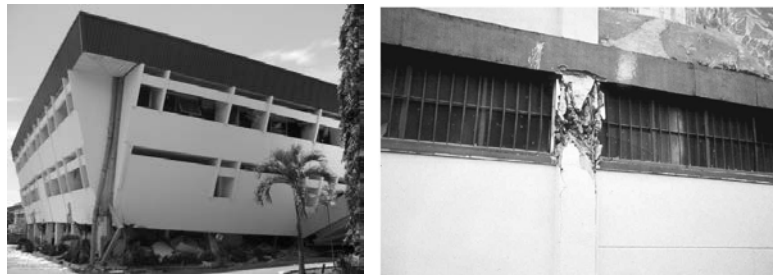
Figure 1 Negative effects of infill panels; soft storey mechanism [2] (left), short column mechanism [3](right)
