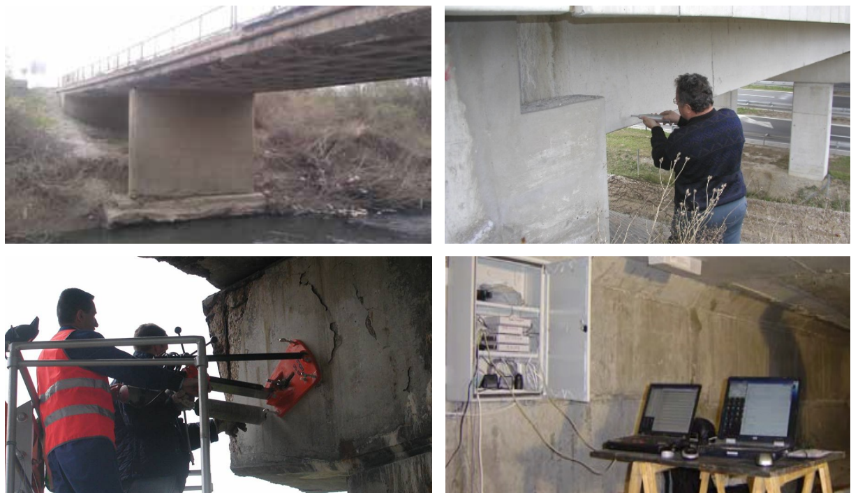
Fig. 16. Main approaches in damage detection: visual inspection, non-destructive testing, probing and structural health monitoring.
