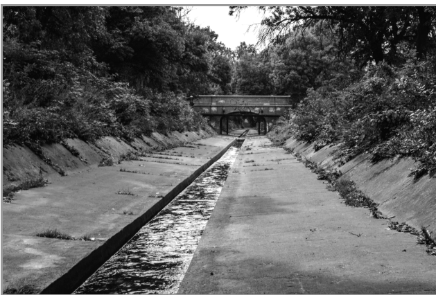
Photo 6. The concrete river channel of the Jasień : the brick bridge in the distance is next to Cieszkowskiego St Photo: J. Jędruszkiewicz
