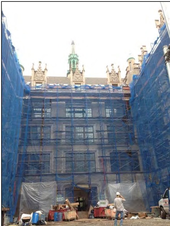
Artspace , a creative process grantee based in East Harlem, creates, fosters, and preserves affordable spaces for artists and arts organizations. Above, an abandoned public school building, P.S. 109 in the El Barrio section of Harlem, is being transformed by Artspace into a vibrant, new, sustainably developed arts facility containing 90 affordable residences for artists and their families, and 12,000 square feet of space for arts.
