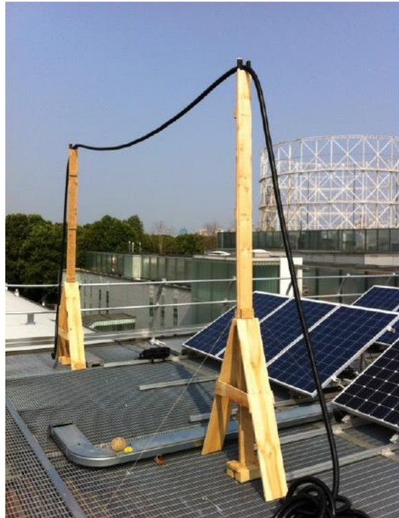
Fig. 4. Structure for simulating medium voltage overhead lines shadowing
