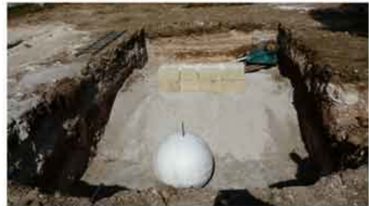
A polystyrene sphere, simulating a cavity, with a tuff wall simulating a foundation
