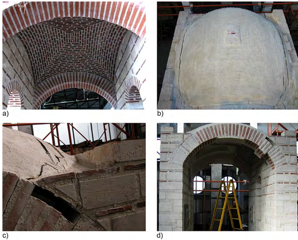
Figure 2-37. Cross vault tested in NTUA, Athens: a) interior view of the cross vault tested in NTUA; b-c-d) damages at the end of the test
