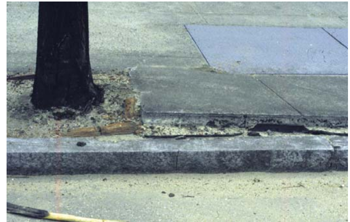
Tree roots can cause hazardous conditions, such as ? sidewalks.
