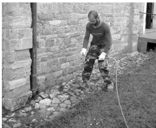
Fig. 1. Flaming on the external perimeter of the Basilica of San Piero.
