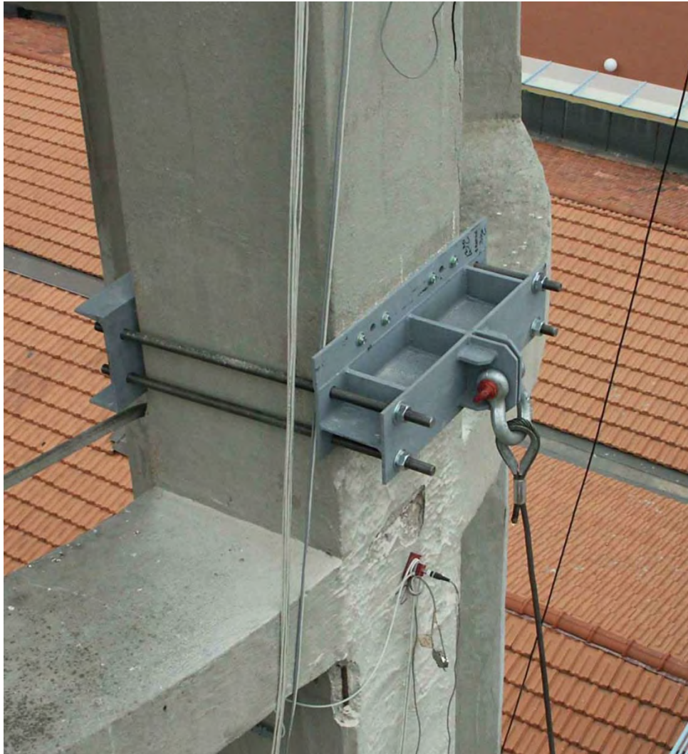
Figure 5 Cable attachment on the structure
