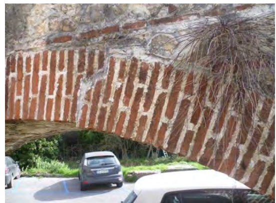
Arch n. 22 – Side A Relative displacement in the mortar joint plane
