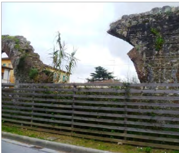
Figure 21 Arch nr. 99, collapsed
