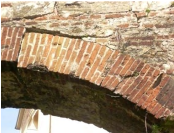
Arch n. 101 – Side A Relative displacement in the mortar joint plane
