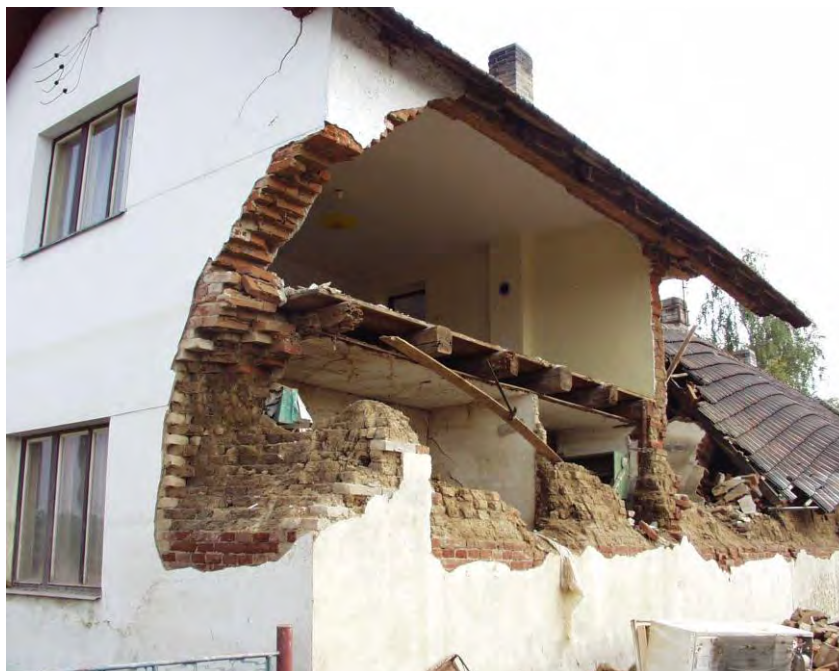
Figure 6 Partial collapse of a residential house without ring beams.
