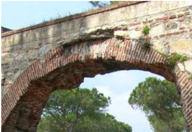
Arch n. 163 – Side A Deterioration of arch's bricks at the extrados and intrados, caused by lorry impact
