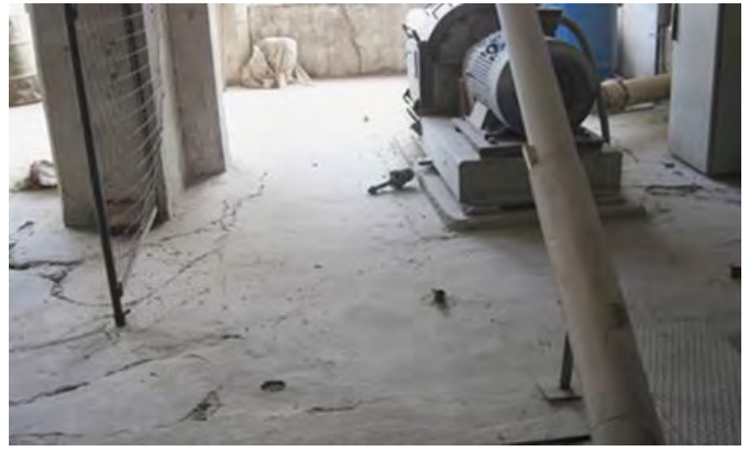
Picture 8: Detail of the flooring. Presence of several patina and relevant not cross cracks
