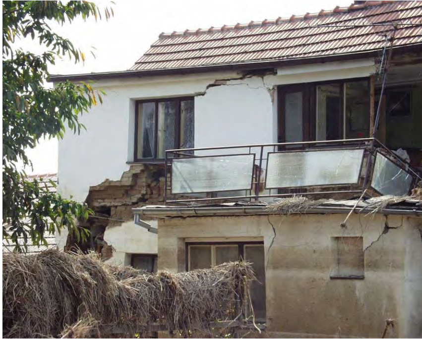
Figure 5 Damaged residential house with insufficient foundation.
