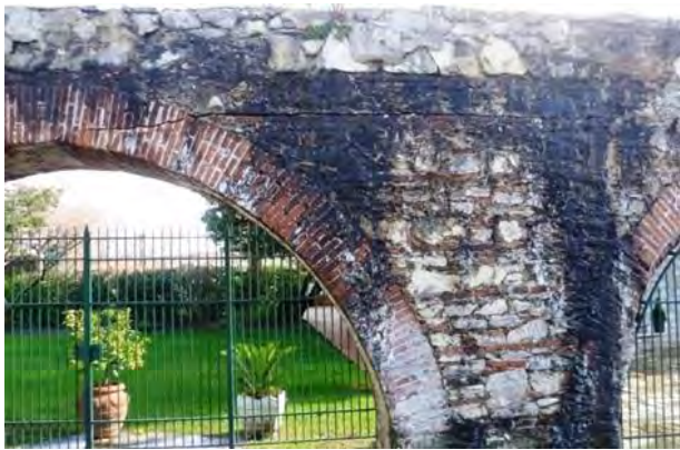
Arch n. 16, 17 – Side A Vertical settlement appearing by a crack in the backfill, extended to arch's brick
