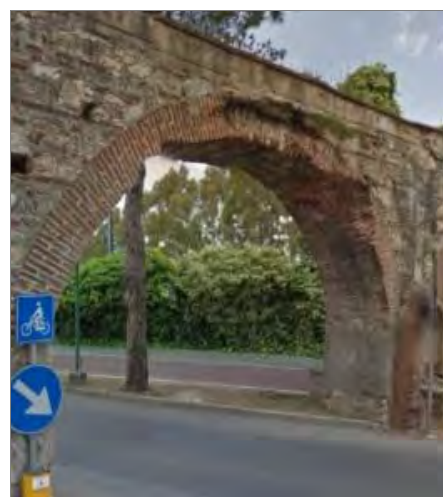
Figure 22 Arch n°162, damaged by vehicles impact
