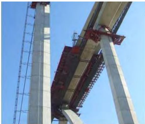
Figure 6 Position of the formwork before the accident
