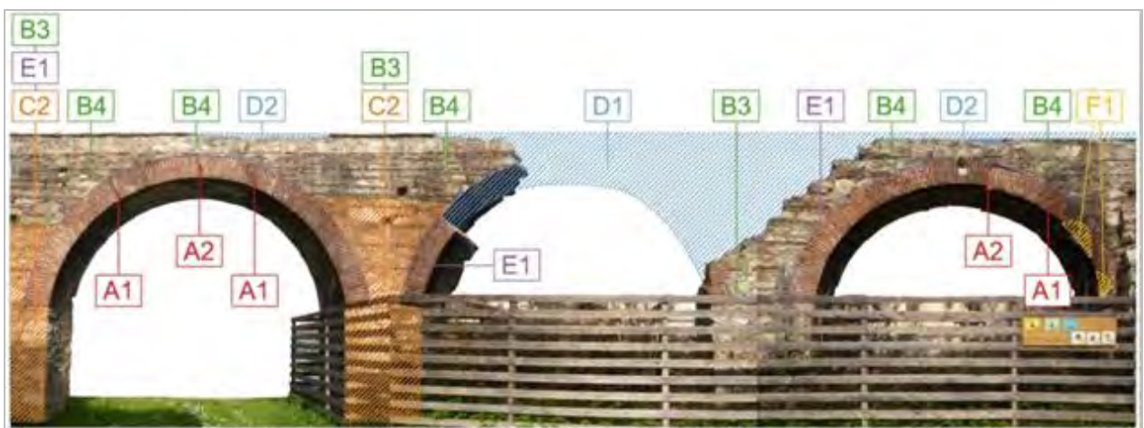
Figure 44 Crack pattern of arches n. 98, 99 and 100 – side B
