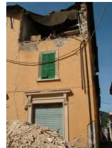
Figure D.2 Out of plane overturned wall
