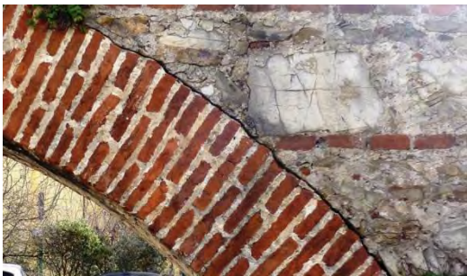
Arch n. 113 – Side B Detachment between the arch's bricks and the backfill.
