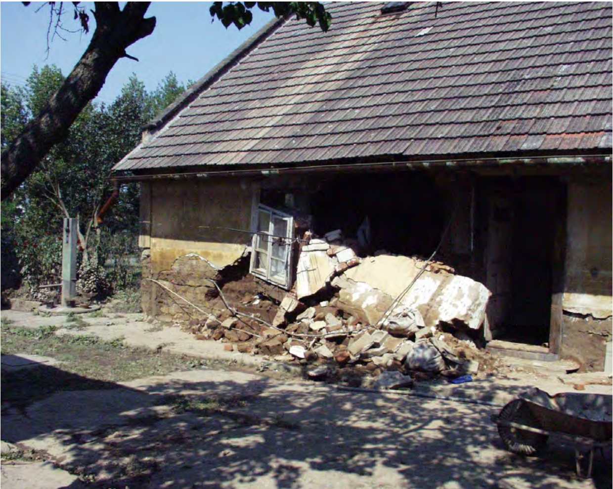
Figure 7 Failure of a structure with unfired masonry units.
