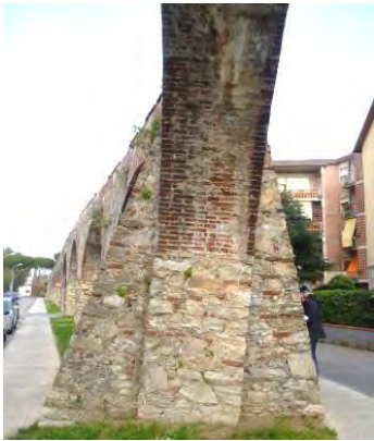
Arch n. 144 – Section Out of plane rotation (9°) of a pillar between buttresses
