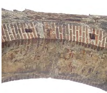
Arch n. 137 – Side A Detachment of some brick elements from the arch
