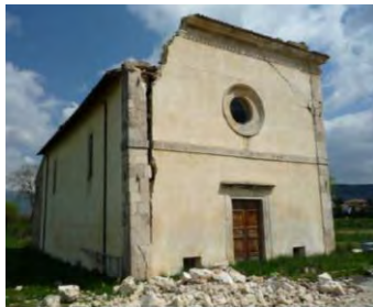
Figure D.1 Overturned tympanum and cracks indicating incipient overturning of the building facade
