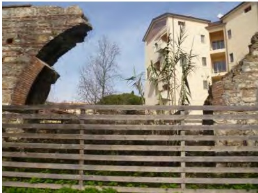
Arch n. 100 – Side B Total collapse of the arch
