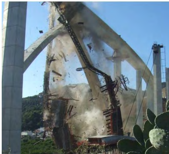
Figure 4 Collapse of the MSS (photograph: F. Nederlof)
