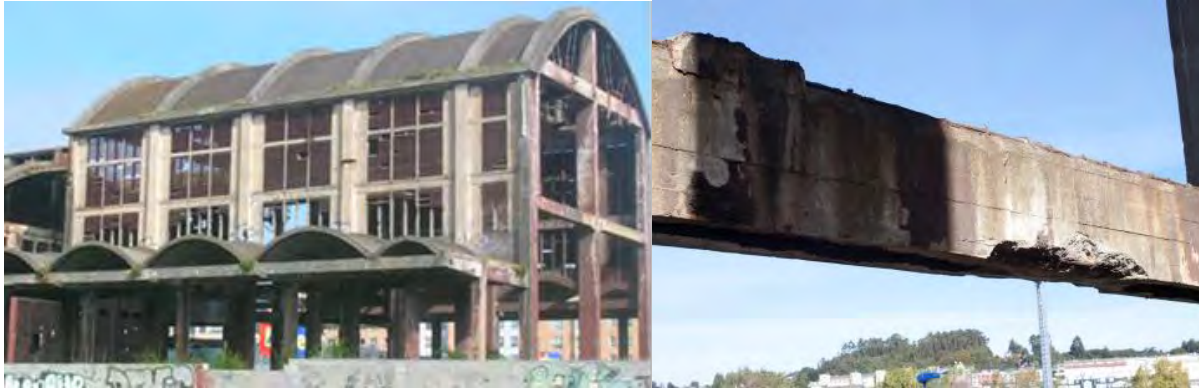
Figure 1 Existing industrial building before the transformation and one of the beams affected by corrosion
