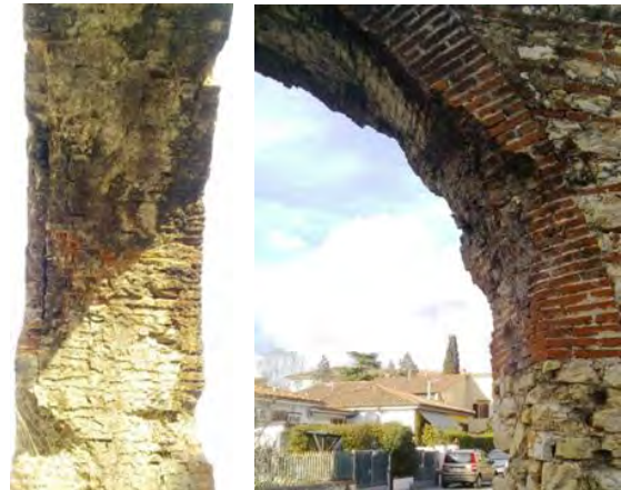
Arch n. 163 – Side A Deterioration at the intrados of the arch and deterioration of the façade of the arch
