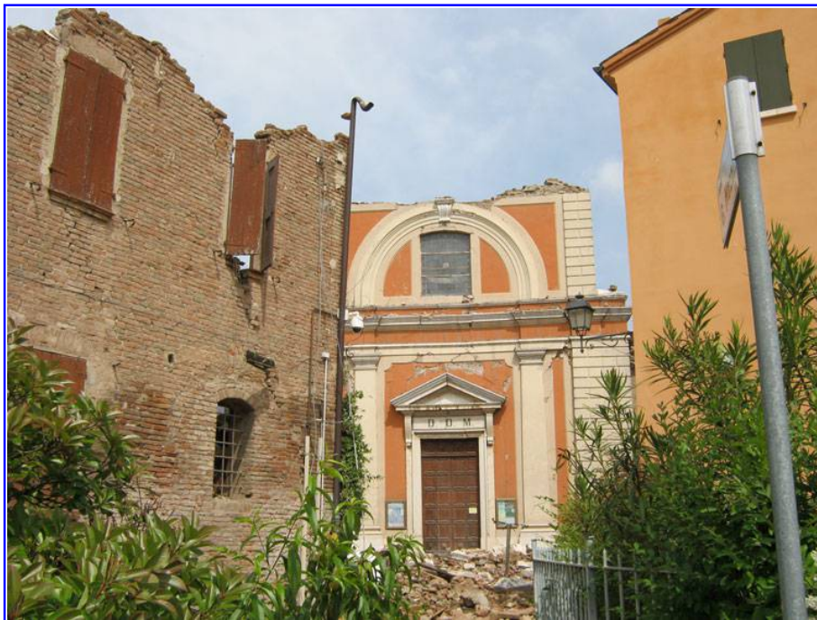
FIG. 1. Parish Church of XVII century destroyed by the earthquake. City of San Felice (Modena).
