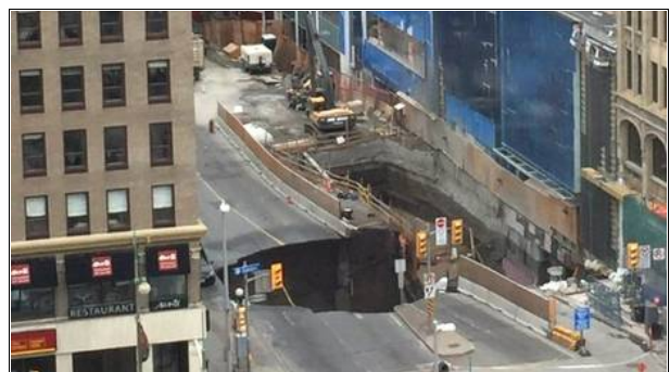
Figure 7. Sinkhole in Ottawa (Canada) (source: http://www.theglobeandmail.com/news/national/gaping
