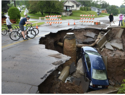
Floodwater caused this one in Duluth. (Brian Peterson/Star Tribune/Associated Press)
