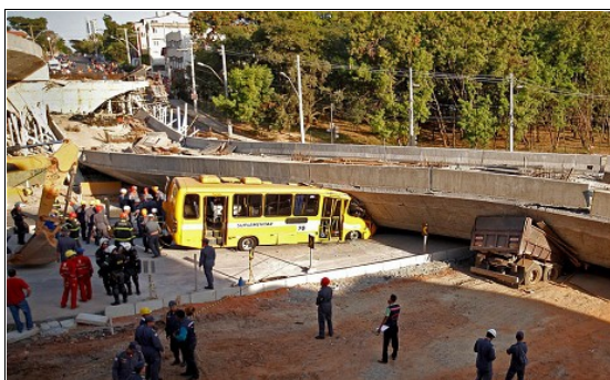
Figure 6. Collapse of a viaduct under construction in Belo Horizonte (Brazil) (source:
