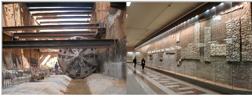
Figure 68. Interferences with excavations for building underground – Caracas underground (on the left), and Athens underground (on the right)
