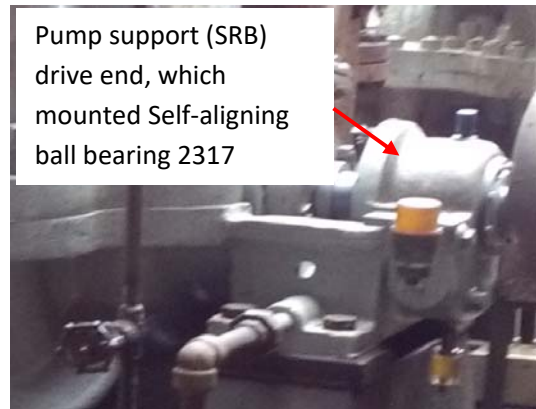
Figure 3.26: Two stage centrifugal pump PS27
