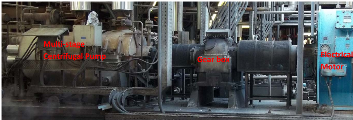
Figure 4.14: Global view of motor , gear box and pump
