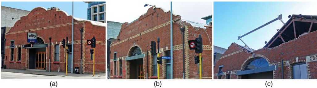
Figure 16. Examples of progressive damage to retrofitted parapet: (a) former Canterbury Horse Bazaar, prior to earthquakes; (b) partial collapse after 22 February 2011 earthquake; (c) parapet and wall collapse after 13 June 2011 earthquake.
