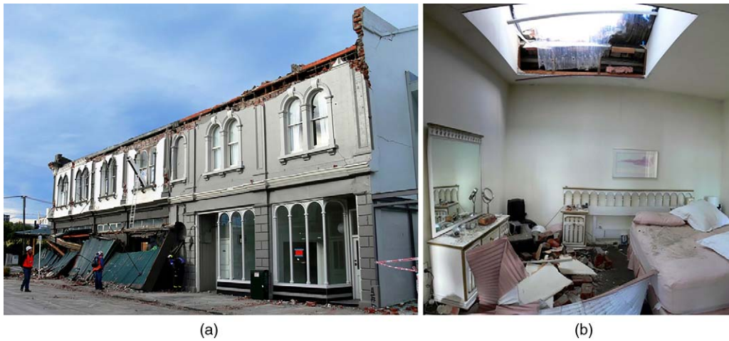
Figure 1. Examples of parapet failures during the 2010/2011 Canterbury earthquakes: (a) URM parapet that has collapsed onto the street frontage; (b) URM parapet that has collapsed into the building interior.
