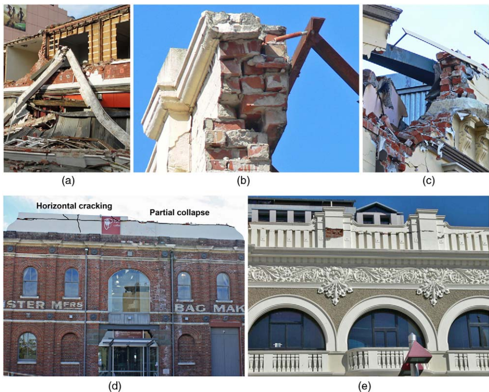
Figure 21. Typical examples of observed failure mode for adopted retrofit interventions: (a) collapsed concrete beam; (b) bracing back to structural element – short embedment of the adhesive anchors; (c) steel strip; (d) bracing back to structural element – cracking above the horizontal steel strip (highlighted in black); (e) steel strip – cracking above the horizontal steel strip.
