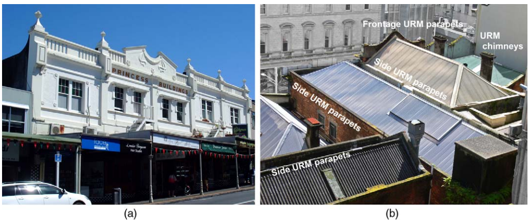
Figure 2. Typical URM buildings with multiple parapets and other nonstructural elements such as chimneys and ornamental pinnacles. Images taken in Auckland, New Zealand: (a) URM parapet on street frontage; (b) rooftop view.
