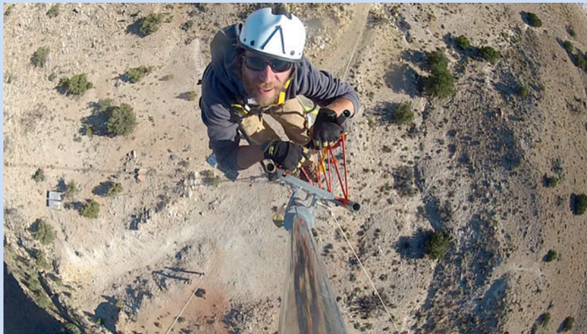
FIG. SBI. NCAR technician Chris Golubieski from ISFS during the construction of the 40-m mast on the south rim of the Meteor Crater. Photo courtesy of Tim Lim.
