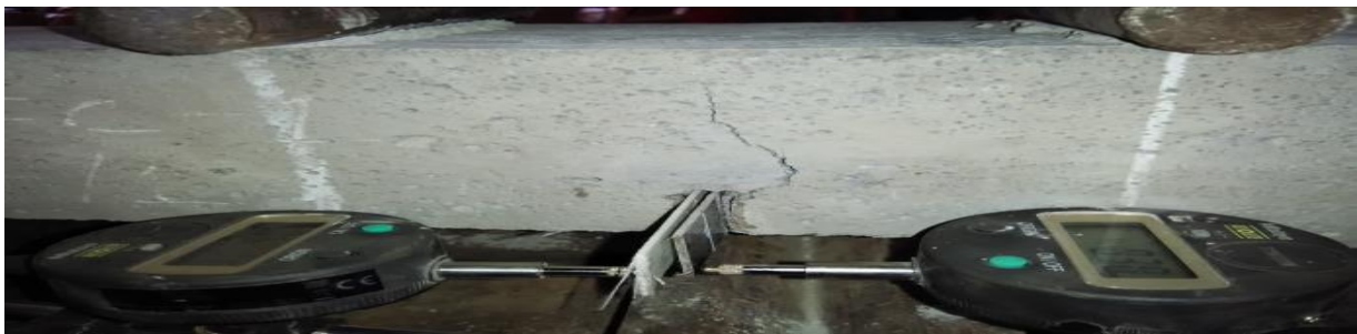
Fig. 4.6.2 Crack Pattern of GFC-1
