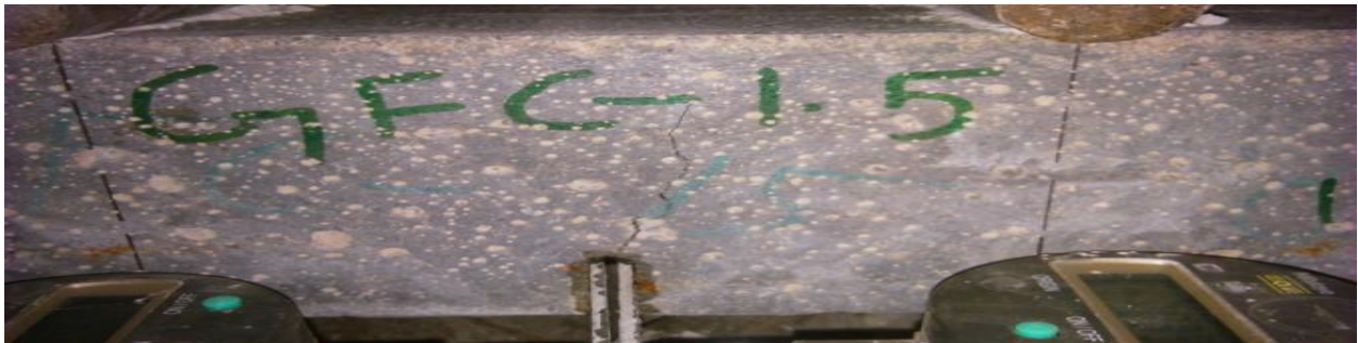
Fig. 4.6.3 Crack Pattern of GFC-1.5
