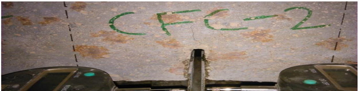
Fig. 4.6.15 Crack Pattern of CFC-2
