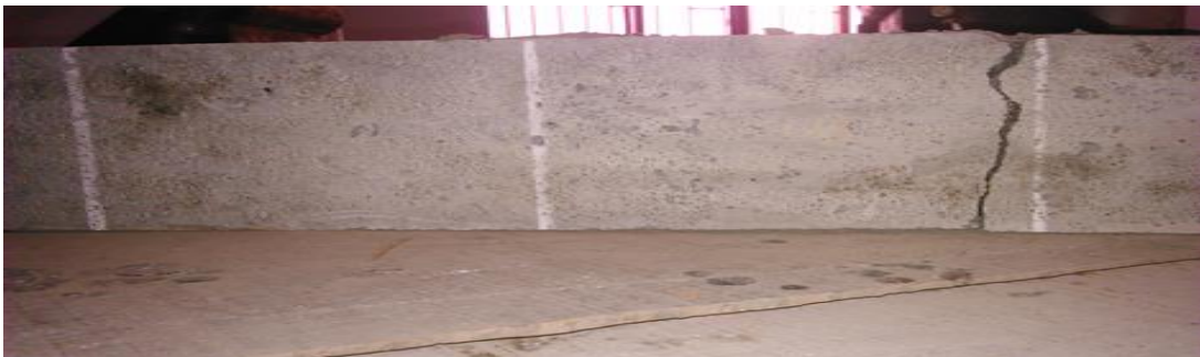
Fig.4.5.1 Crack Pattern of PSC
