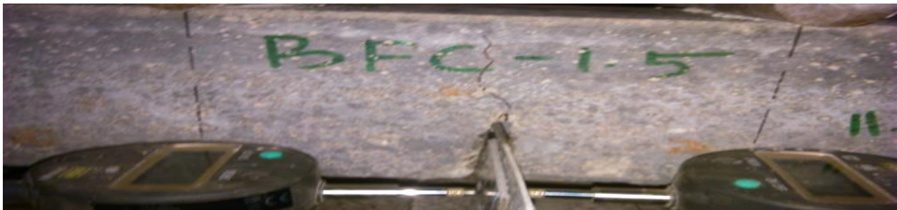
Fig. 4.6.8 Crack Pattern of BFC-1.5
