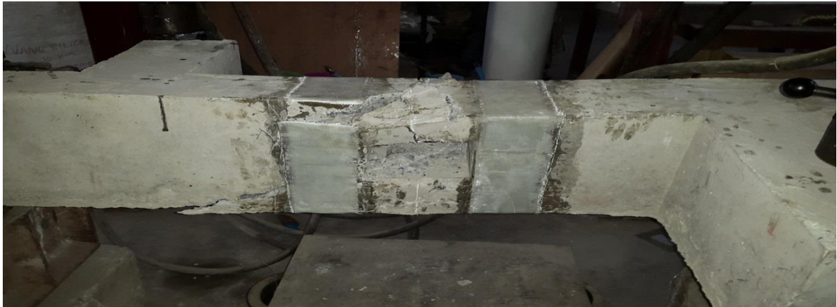
Fig 4.4 Crack pattern in BRO1
