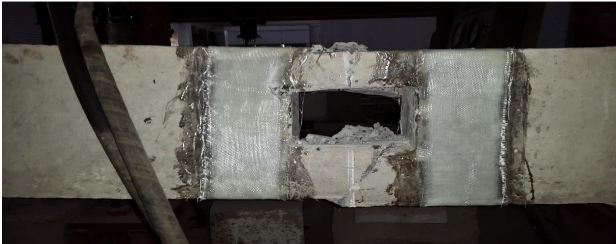
Fig 4.5 Crack pattern of BRO2
