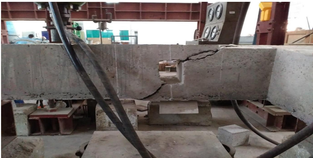
Fig 4.3(b) Crack pattern in BSRO
