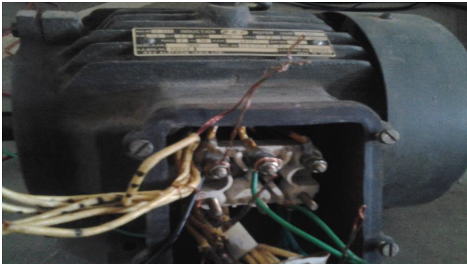
Fig.2.4 Stator Winding Turn 1 to (3N/7) Shorted
