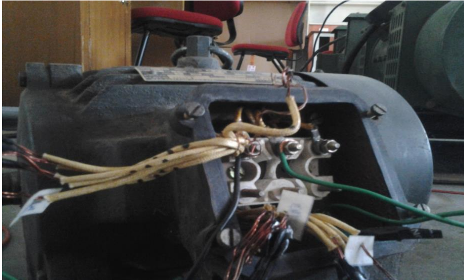
Fig.2.3 Stator Winding Turn 1 to (N/7) Shorted
