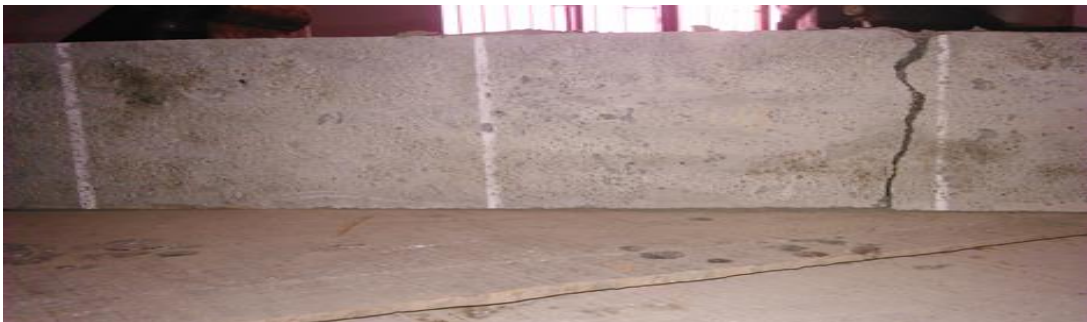
Fig.4.5.1 Crack Pattern of PSC
