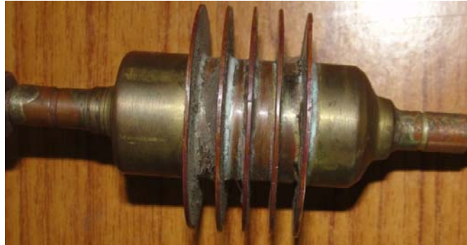
Figure 4.2 Typical pictures of the after cooler
