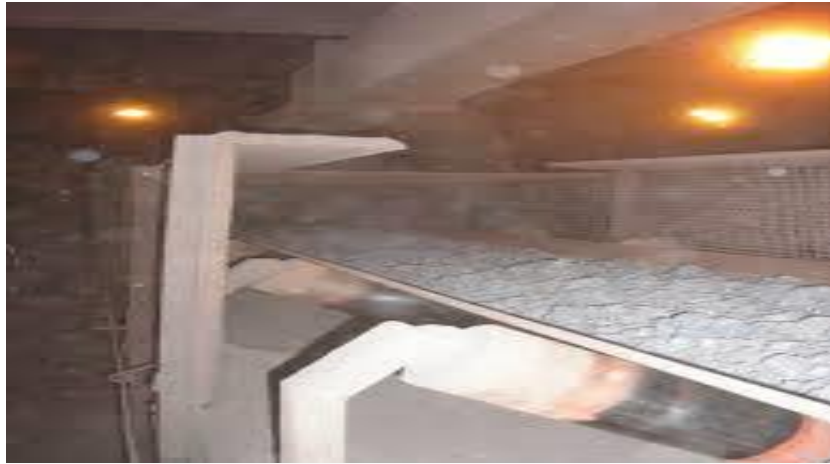
Grilling system for protection of spillage of coal
