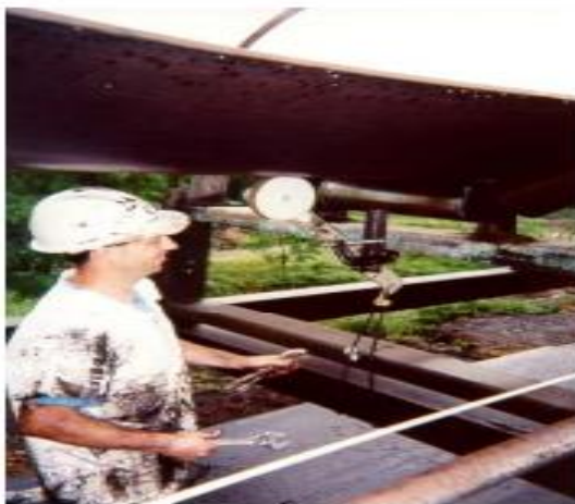
Belt speed monitoring by tachometer installing on carrying side of belt
