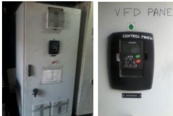
Controlling the long travel speed of stacker/reclaimer by VFD Panel
