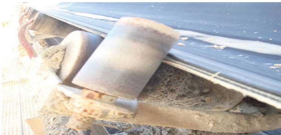
Idler tracking system in BCS
