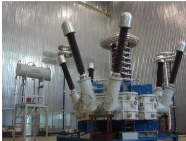
Fig 1.5: Superconducting Fault Current Limiter
