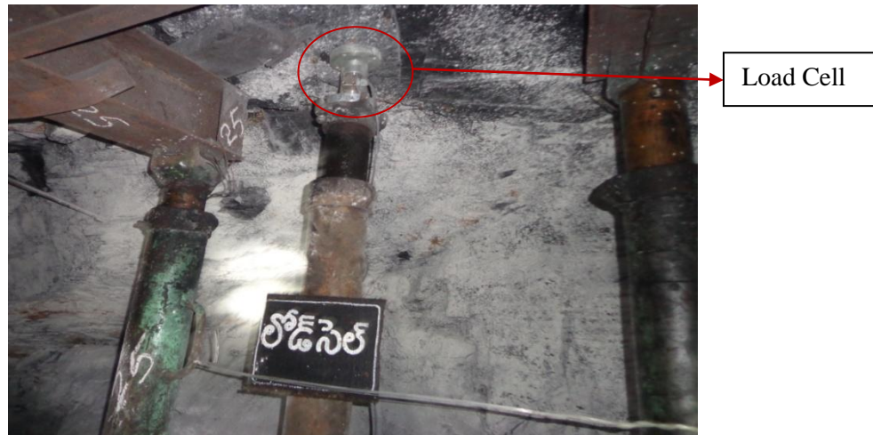
Fig 1.4 VW type load cell installed above a hydraulic prop[3]
