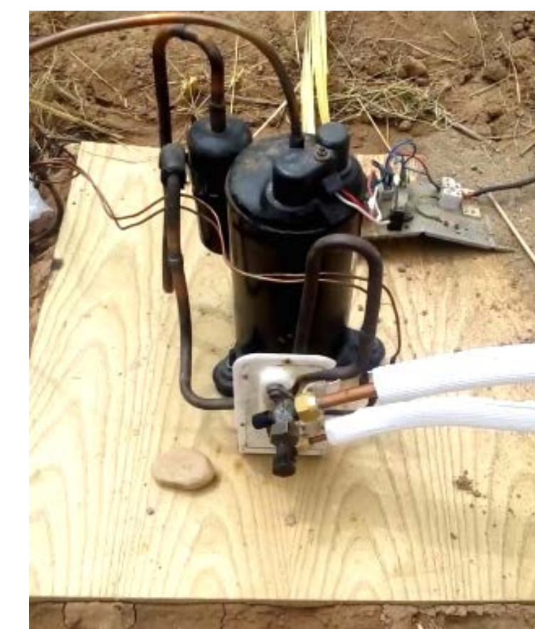
Fig.9 Fully assembled DX geo thermal system
