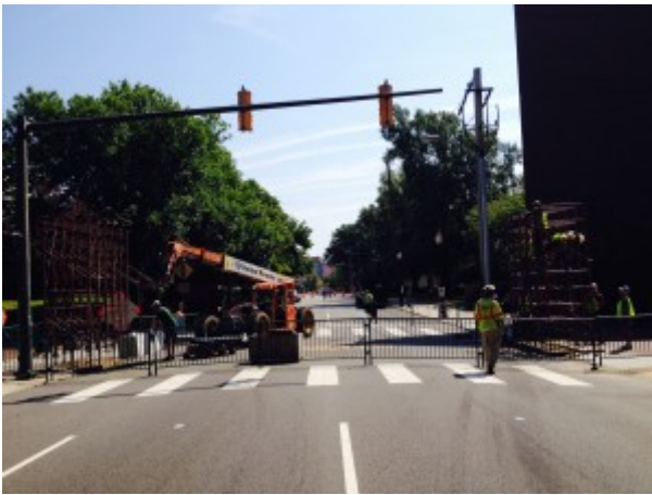
West Main Street is closed to traffic for two days so a pedestrian bridge can be assembled.
