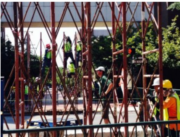
Workers assemble the framework for the pedestrian bridge over West Main Street.
