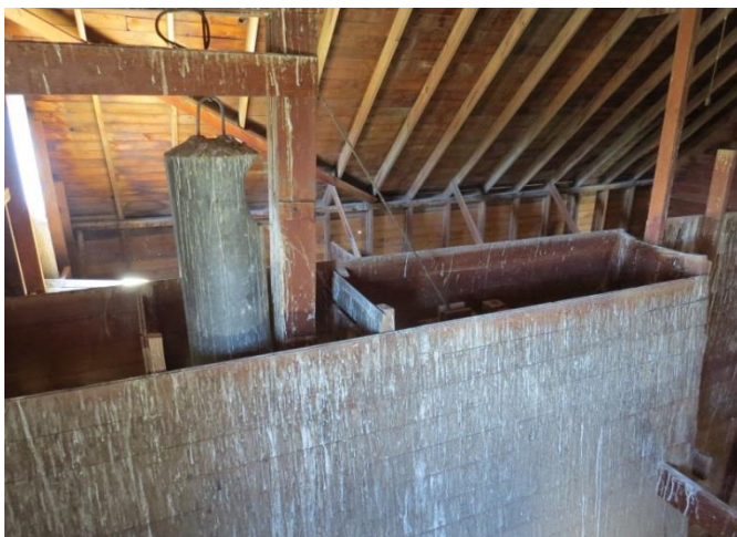
Figure 125. The highest portion of the press at the Gendron Hop Kiln. The counter weight on the left hand side is at the top when the press is fully extended down (see picture of press in down position on main floor in the baling room). (Terri Towner, 2016)
