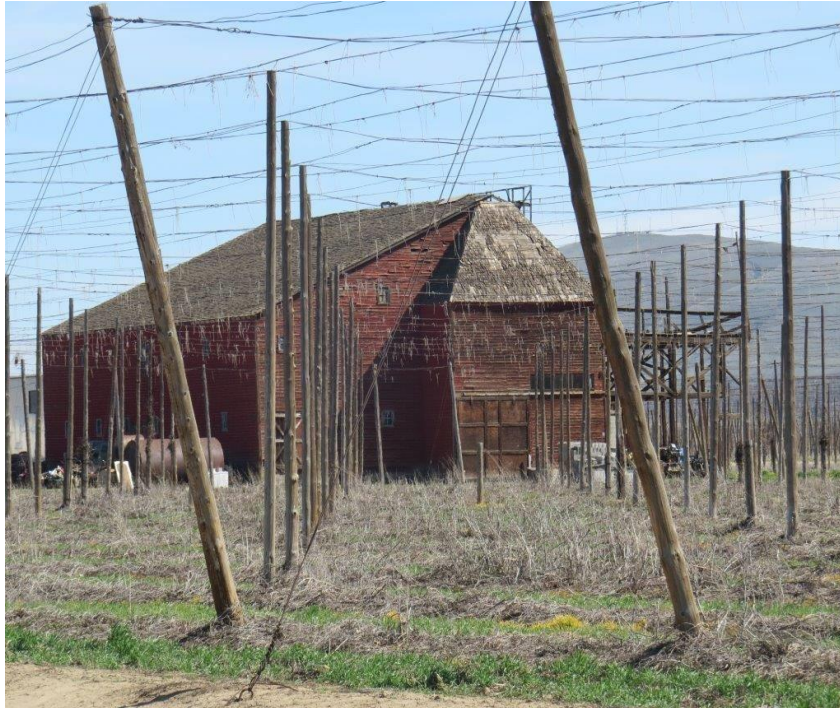
Figure 103. Ovide Brulotte Ranch Kiln on Bell Road near Moxee. The deck that faces south is in disrepair and the roof needs to be replaced, but the internal condition of the building is in very good shape. Boasting four separate kilns that were heated with heating oil or propane. It had a conveyor system that moved hops from one place to another. It is just down Bell Rd. from the Gendron Ranch Kiln. (Terri Towner, 2016)
