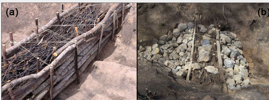
Fig. 8 - Construction process of the rock and biomass mixed dam. Trench constructed and filled with debris from the silvicultural works (a) and reinforced by rocks (b).
