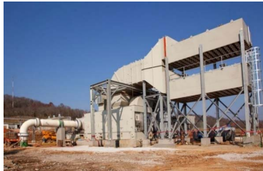
Figure 5: Gas Turbine Filter House
