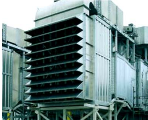
Figure 7: Weather Hood on inlet Filtration System
