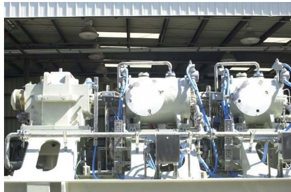
Figure 19: Centrifugal Compressors for Re-Injection Duty at 240 bar (3,500 psi) Discharge Pressure
