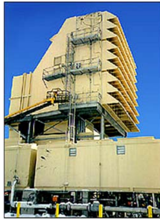
Figure 6: Gas Turbine Filter House
