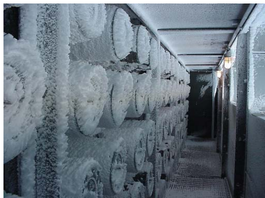
Figure 8: Cartridge Filters with Frost Buildup Due to Cooling Tower Drift
