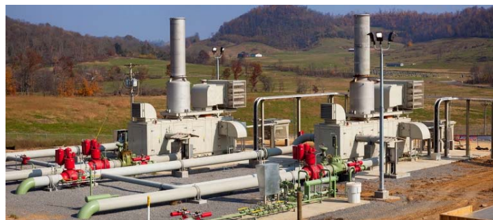
Figure 3: Fully Enclosed Gas Turbine Installation
