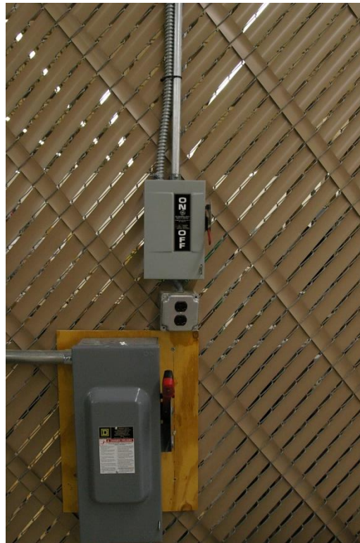
Figure A-11: Cut-off for 3-phase AC for the 50V supplies at top. The bottom cut-off powers the 40cm equipment, do NOT power this off. Located on fence behind the 40cm magnet.
