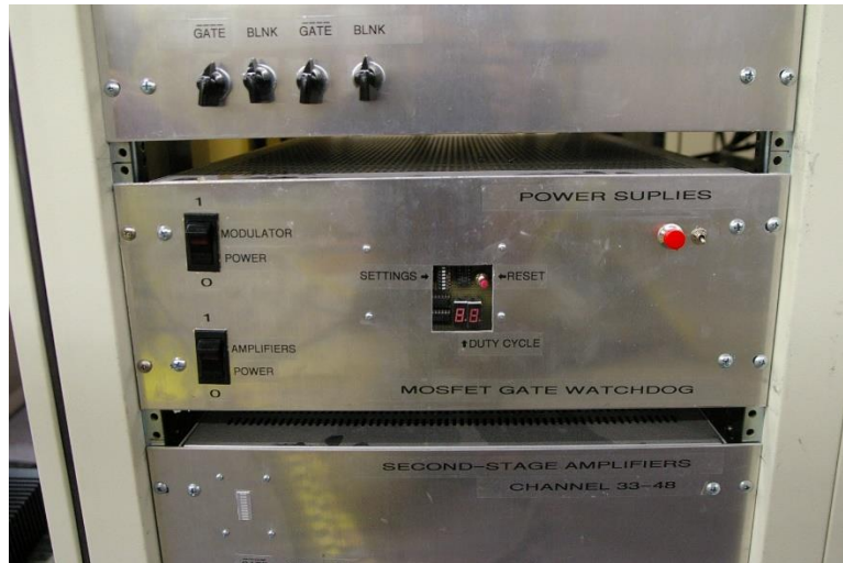
Figure A-10: Low voltage DC supplies for the 64 channel transmitter. Turn on the rocker switch labeled "MODULATOR POWER" first, then the one labeled "AMPLIFIERS POWER". Duty cycle monitor in center should settle to 00 before continuing.
