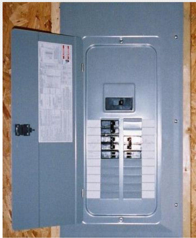
Certificate on Electrical Panel
