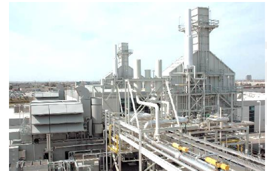
Central Utilities Plant (CUP)
