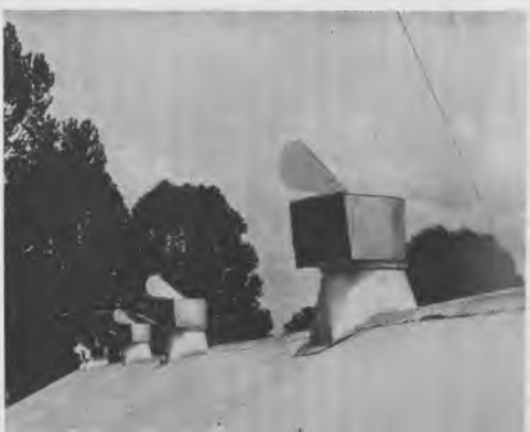
Fig. 5. Another type of ventilator used in the gable type roof.
